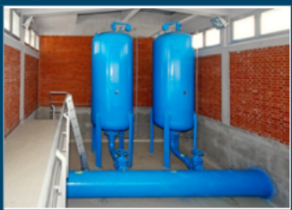
Figure 2 Two vertical air receivers
